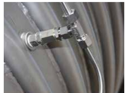
Cleaning nozzles in the outer wall of the tank
